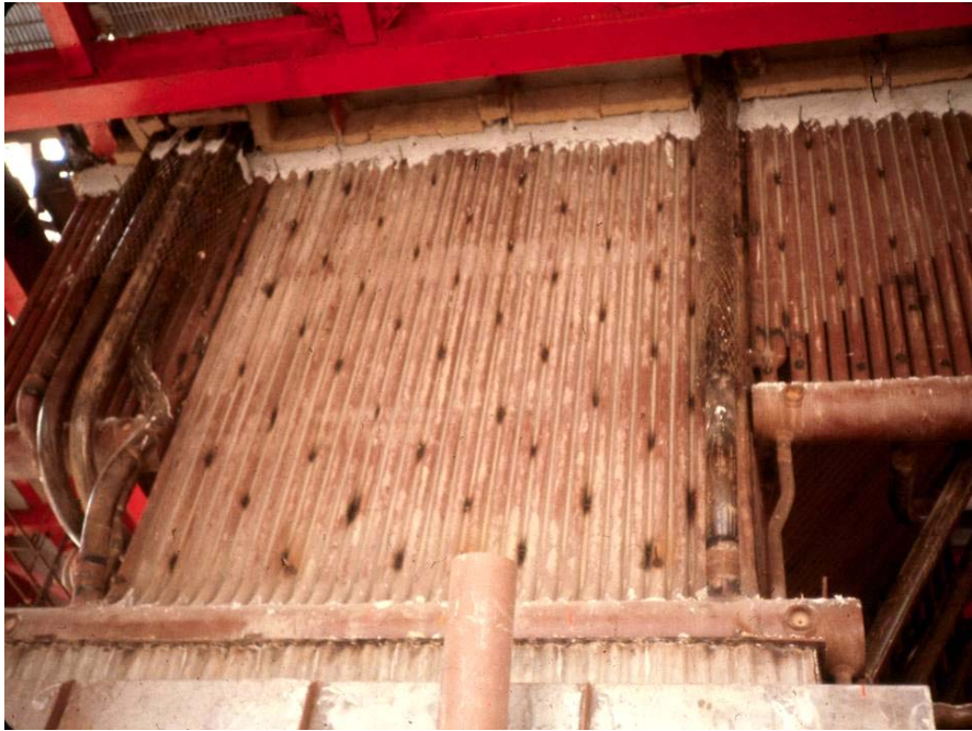
Figure B-1. Waterwall Furnace Section 3
